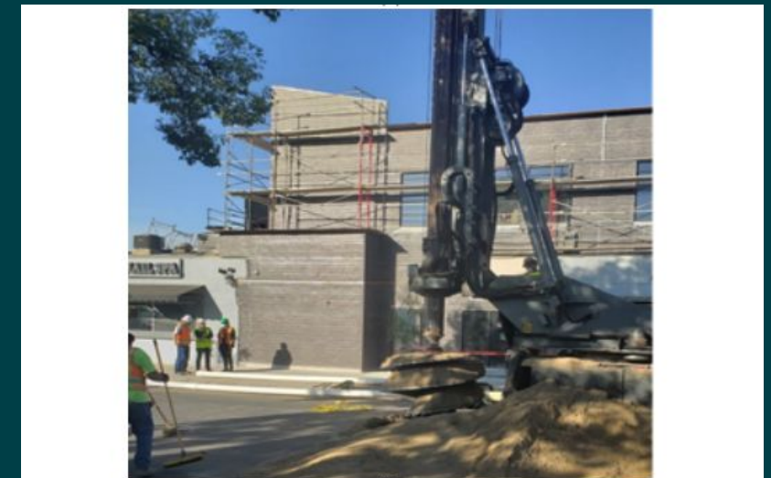
Fig. 1. Drywell system (a). Typical Torrents Maxwell plus® drywell system with sedimentation compartment, (b). Field installation of a drywell
