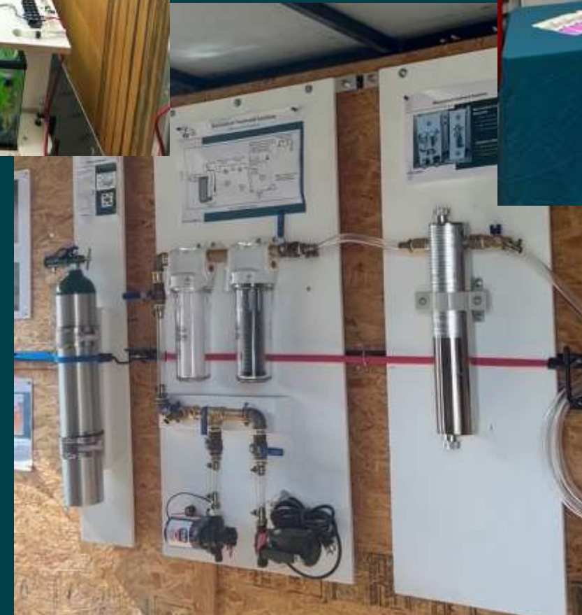
Station 4 – Mechanical Treatment Systems
